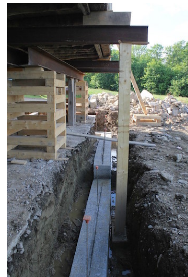
PTF building a frost wall under a raised barn, similar to our foundation project (see their blog for details).
