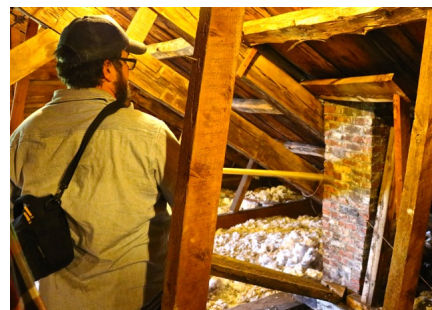
Ed Bell highlighting water damage for the Facilities Board, 6/24/15.
